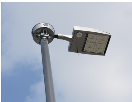
New Light Pole with HUB and LED Fixtures
