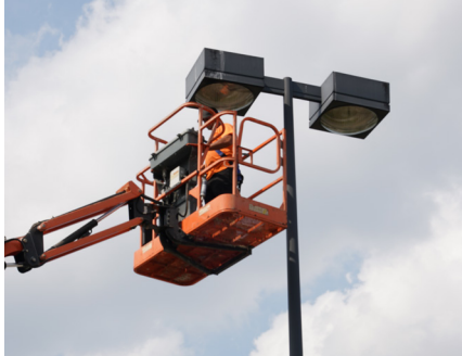
Existing Outdated Parking Lot Light Pole
