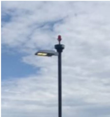
HUB with new LED Fixture &amp; Airport Beacon Light
